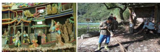
Fig. 20 Maintenance of cultural heritage site and restoration of the Jiang Family Temple in Beipu, Hsinchu
