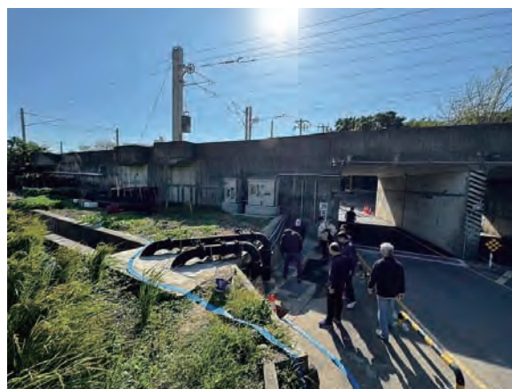
A Complete Flood Prevention System
