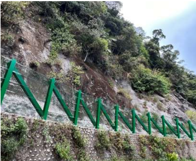
Rock fall prevention fences on the reservoir slopes
