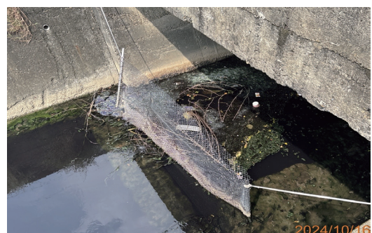
Accumulation of Garbage at River Surface Trash Interception Nets
