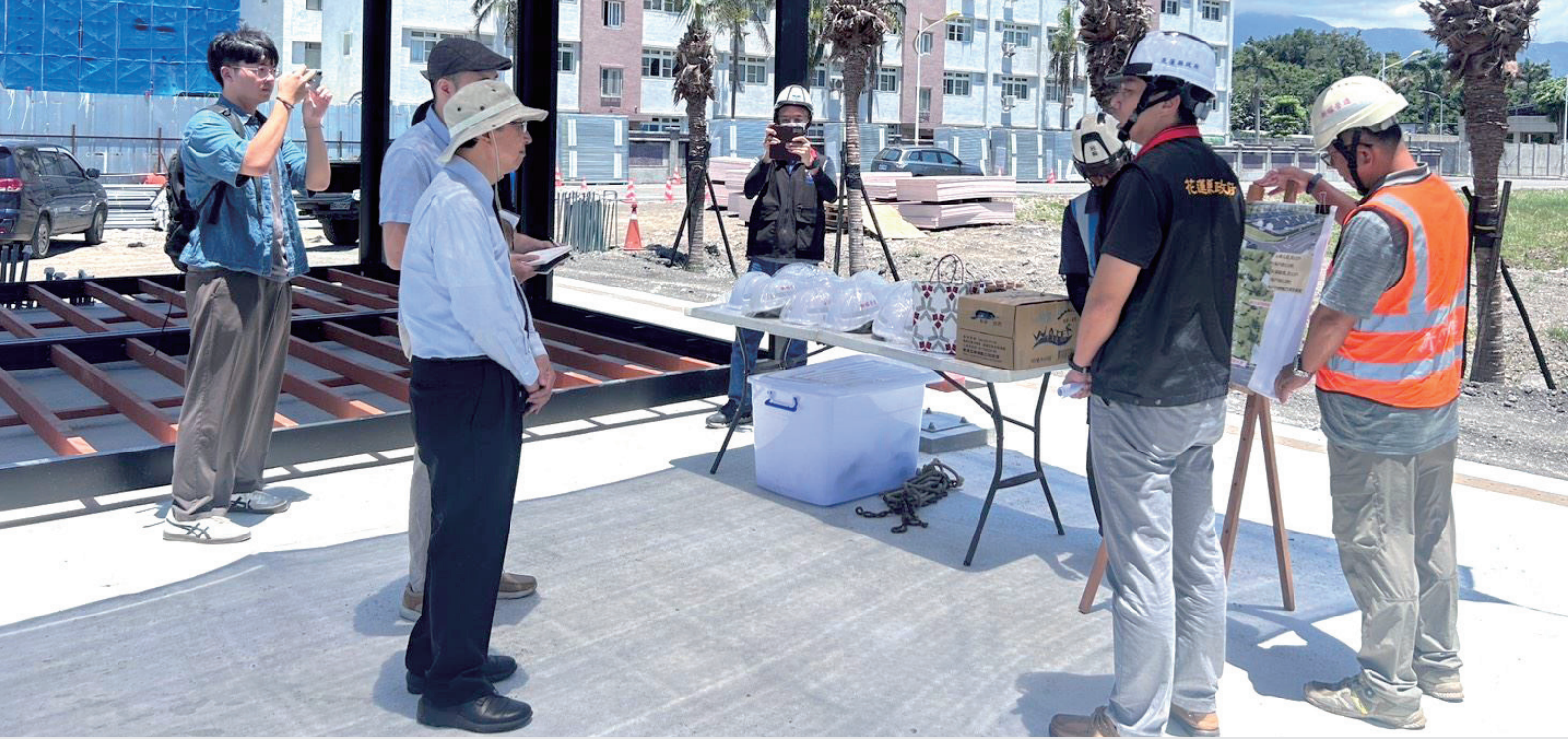
日本防災專家參訪美崙中繼屋施工現場，交流震災重建與中繼住房經驗 Japanese disaster-prevention experts visit the Meilun transitional housing site to exchange post-earthquake reconstruction and housing practices.
