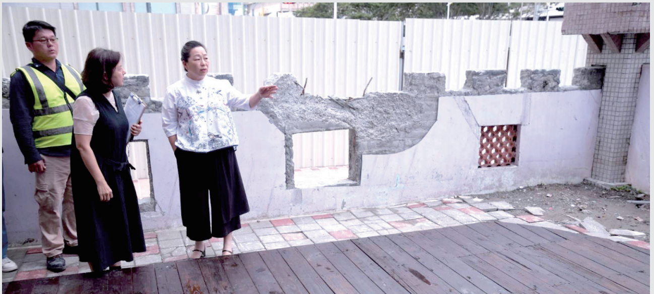
花蓮縣長徐榛蔚視察明禮國小附設幼兒園 0403 地震災損復建工程 Inspection of 0403 Earthquake Reconstruction Project-Mingli Elementary School Kindergarten
