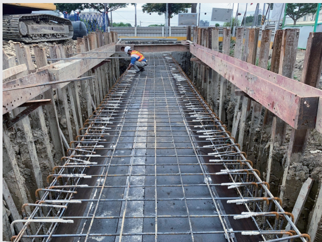
▲ Storm Sewer Project in Minsheng Street, Tanzi District
