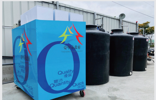
▲ Water purification facilities of Q-WATER
