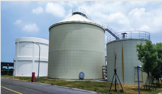
▲ Anaerobic equipment of WaiPu green energy ecological park
