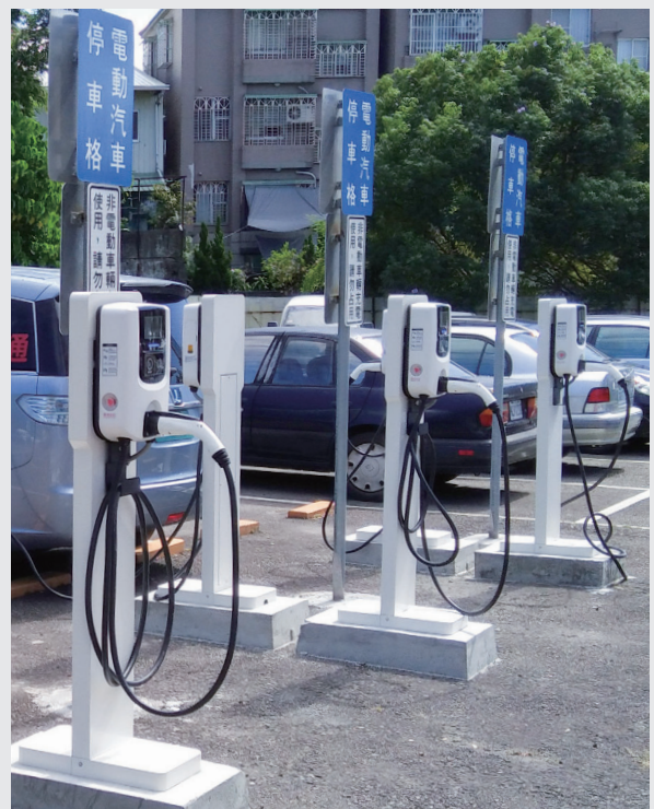
▲ Electric vehicle charging equipment in the second parking lot of Yangming building
