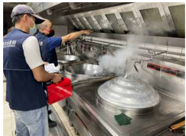
Technical instrumentation to confirm front-end hood performance
