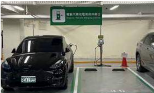
City installed charging station at Revenue Service Bureau
