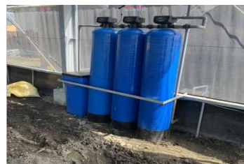
Water quality filtration system
