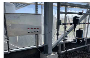
Greenhouse environmental control system
